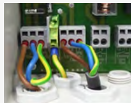
Power supply for the system 1; 2; 3
