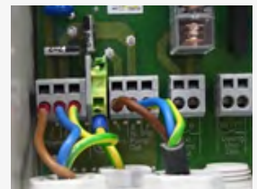
Power supply for the pump 5; 6; 7
